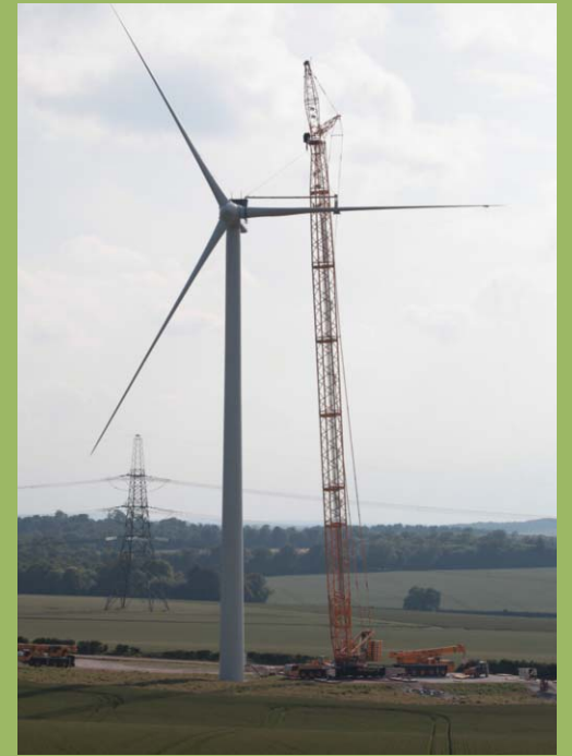
4. Once final checks are completed, the turbine is ready to generate renewable electricity.
